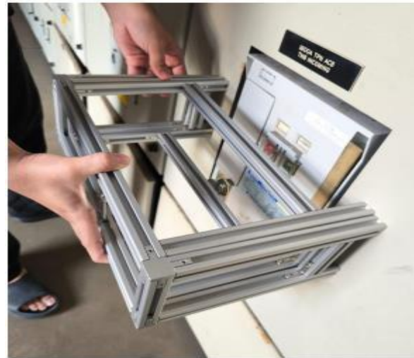
Figure 2.2 Frame at the board panel
